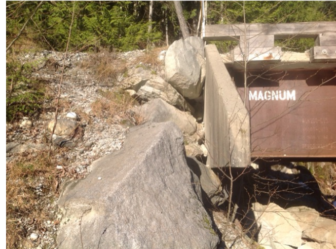
eroded fill right downstream approach
