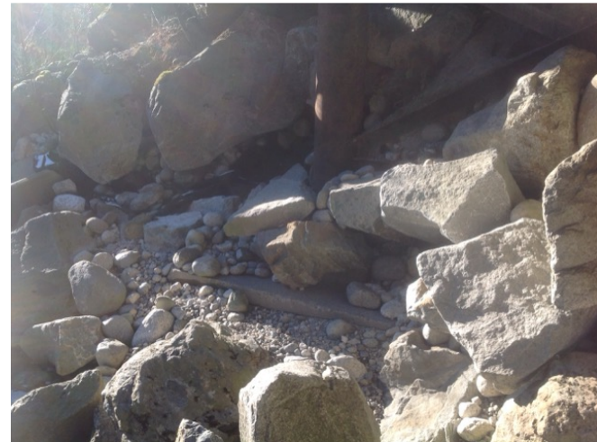
scoured right downstream footing
