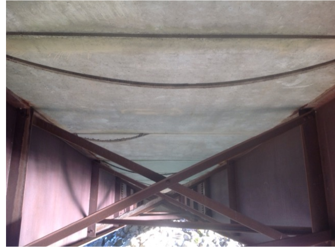
rubber deck seals falling out
