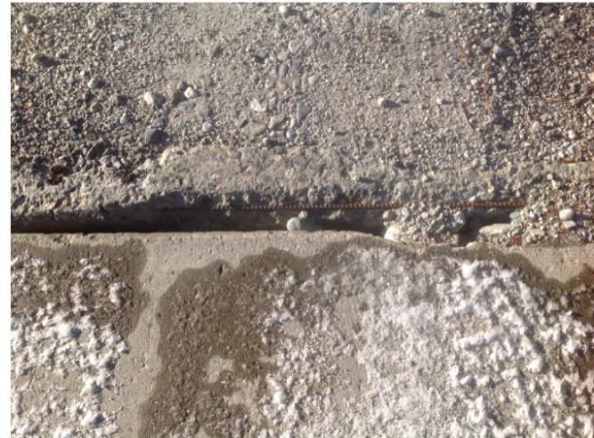
right ballast wall damage
